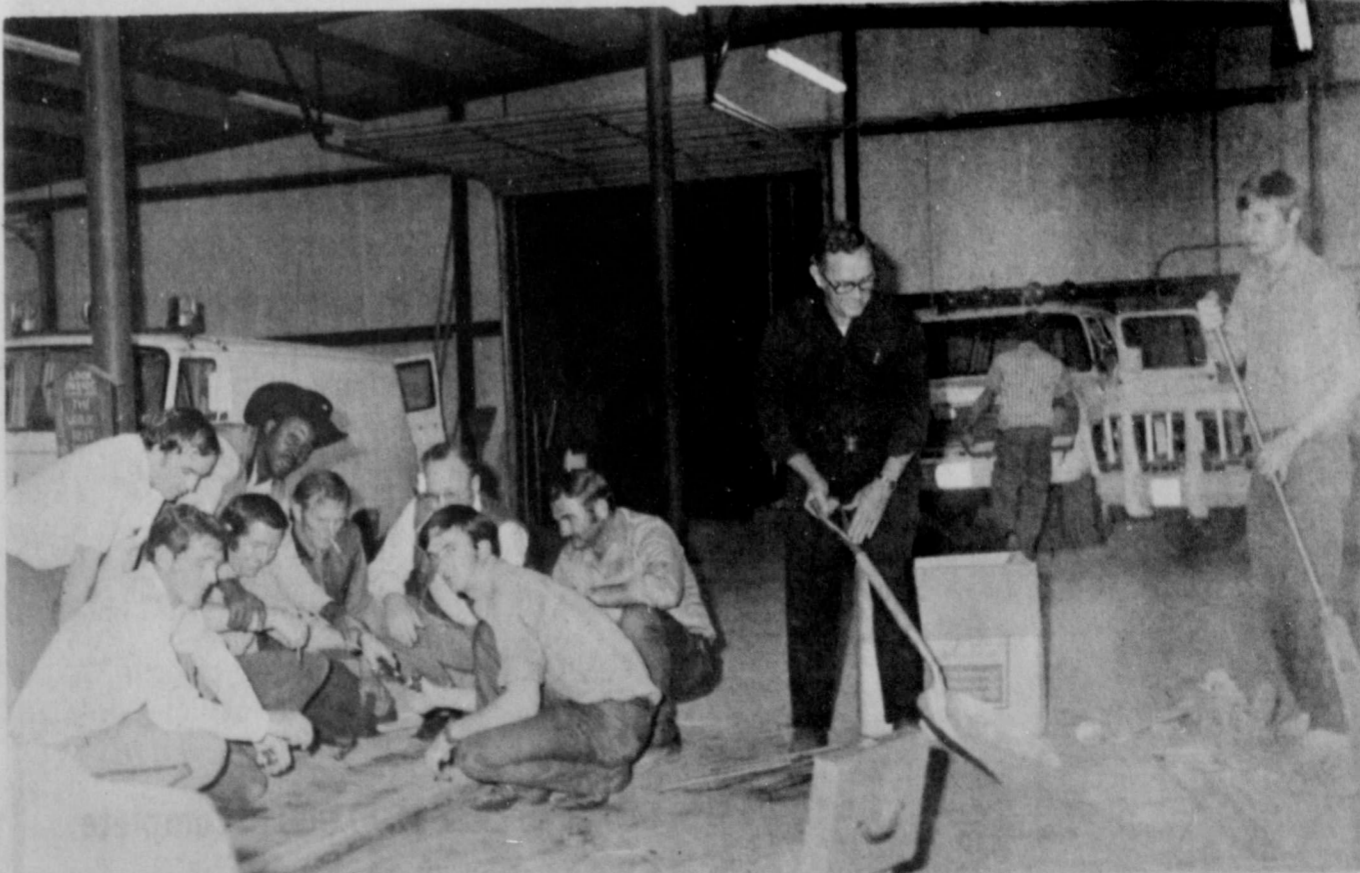
LAST MINUTE CLEAN-UP — Floydada Volunteer Firemen are pictured making a last minute sweep up and building the last part of the kitchen cabinet before the Open House Showing of the new Fire Department building Saturday, November 23. . . . 10 a.m. to 4 p.m. (Staff Photo)
