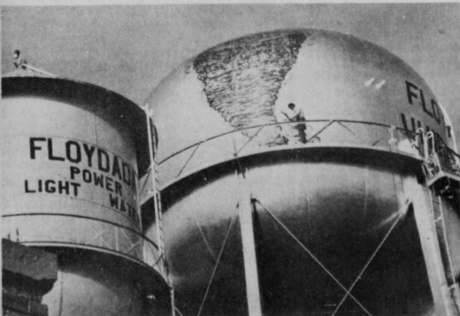
THE CITY OF FLOYDADA'S BIG WATER TANK gets a new coat of paint, complete with "Floydada Whirlwinds" lettering and a big Whirlwind. (Staff Photo by Jim Huggins)
