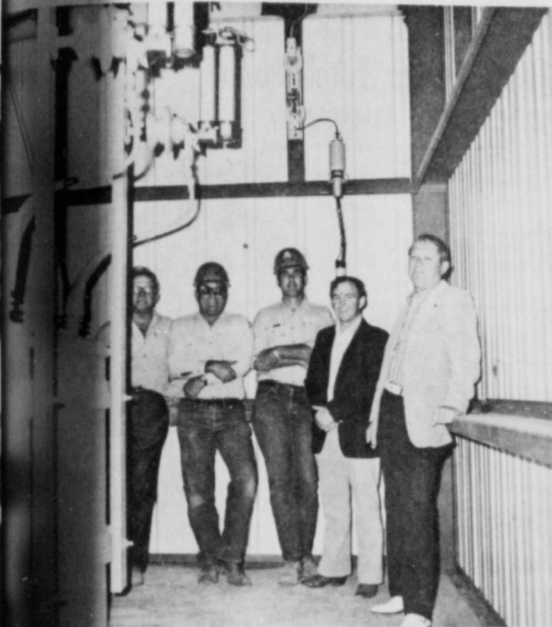
ELECTRIC EMPLOYEES have been working on the new vault for several months. Pictured in the high voltage vault are (left to right) Buddy Bates, Buck Marricle, Dale Anthony Whitfill and Claude Weathersbee. (Staff Photo)
