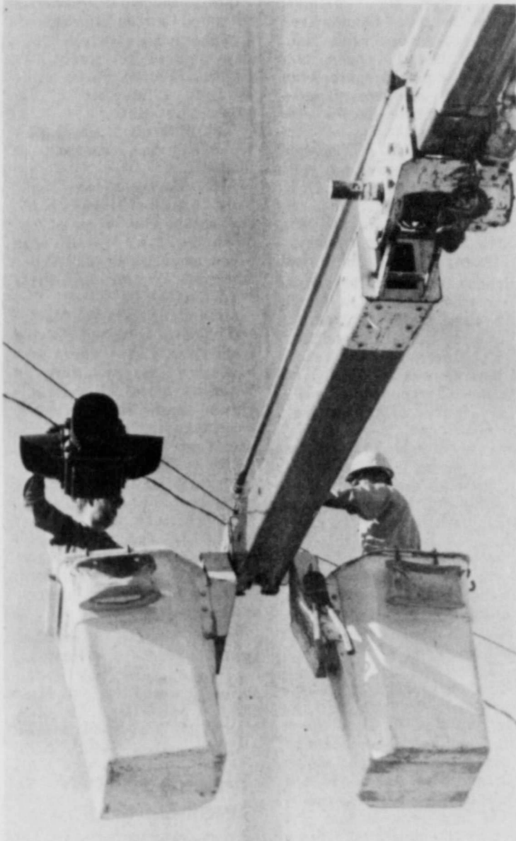
FOUR-WAY STOP SIGNALS — were installed Wednesday on Missouri Street at Main and Wall in Floydada. City workmen Connie Galloway and Tom Simmons are pictured as they put up the signal light at the Main Street intersection. (Staff Photo by Jim Huggins)
