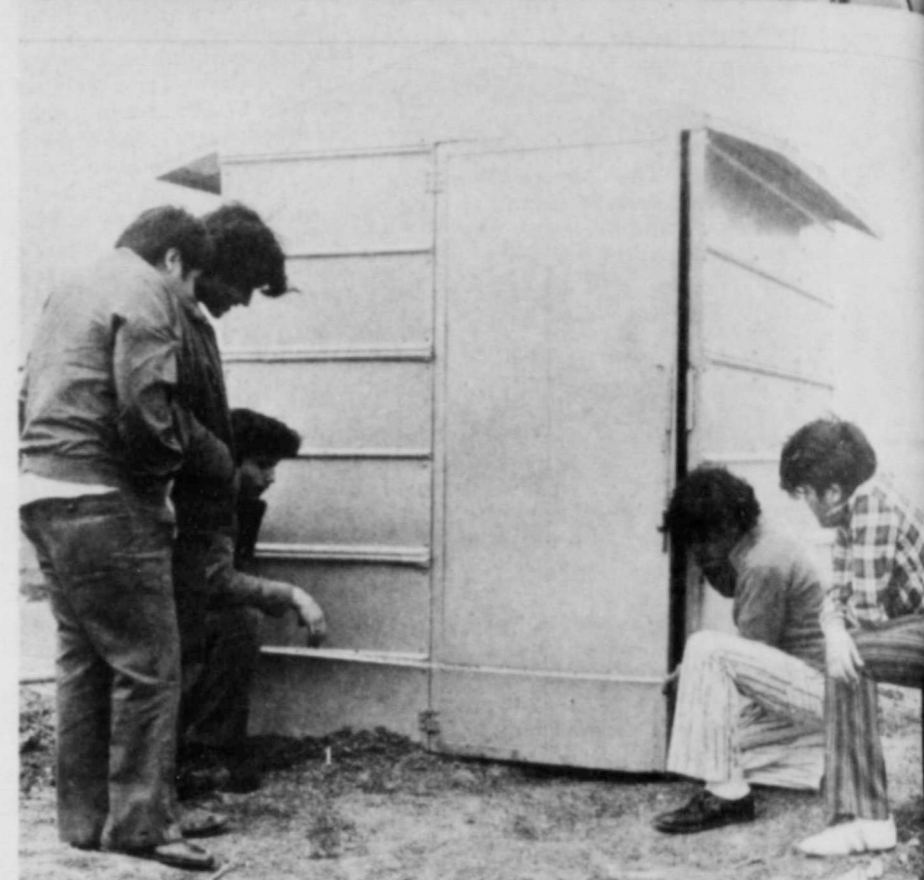
VOCATIONAL RESOURCES STUDENTS... work on a steel building at the class shop at Della Plains School. Pictured left to right in the top photo are Irlas, Ricky Mercado, Romero Sanchez, instructor Al Galloway, Mar Armando Rodriguez. In the bottom picture, the class inspects a building use on a farm near Floydada. (Staff Photo by...)
