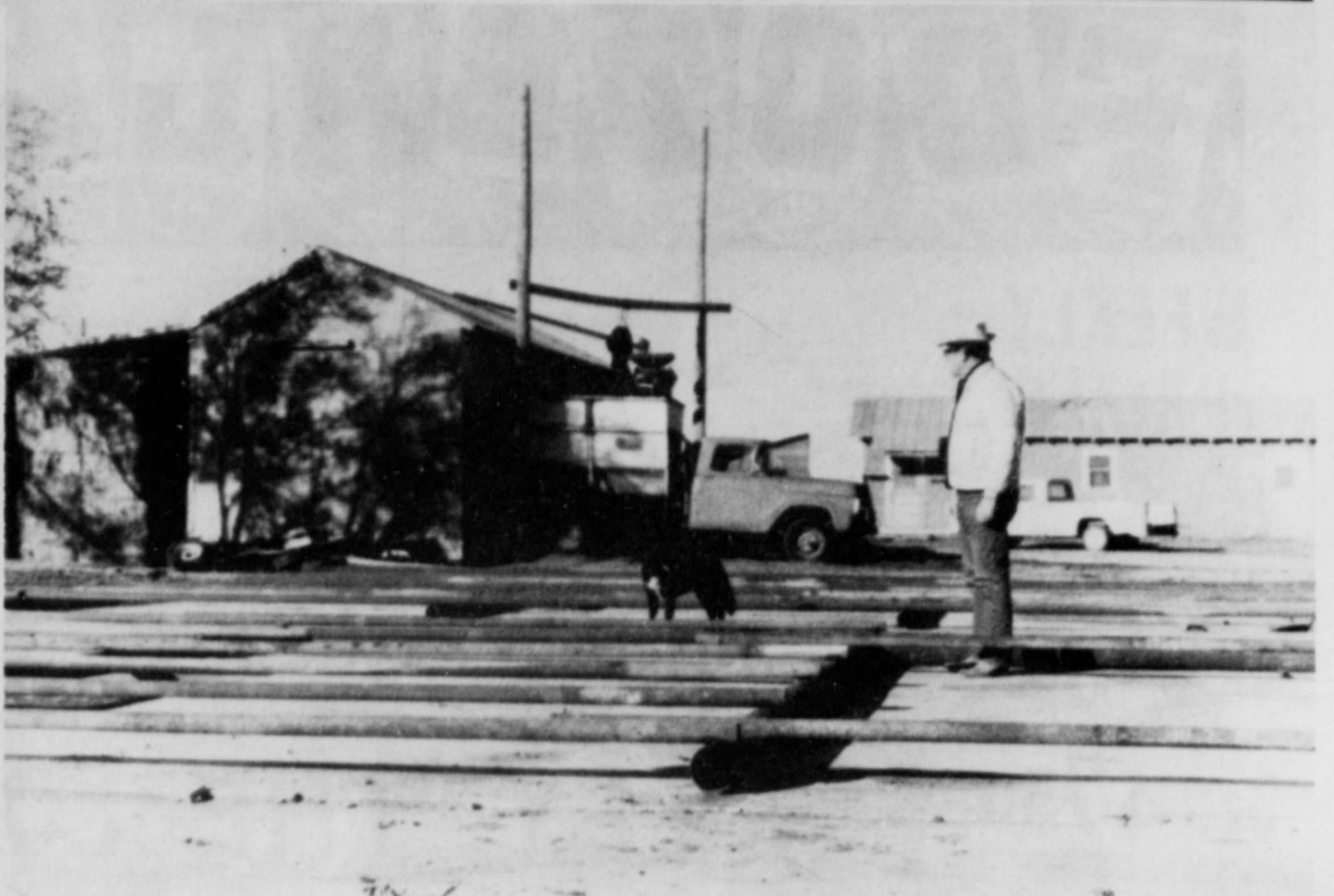
FLOOR FOR NEW FEED building has been poured and steel framing is ready to go up. Old feed barn is in background. (Staff Photo)
