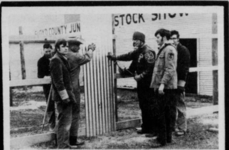
AG IV CLASS...helps with a community service project, building the 60 x 80 extension to the Floyd County Stock Show barn. (Staff Photo)
