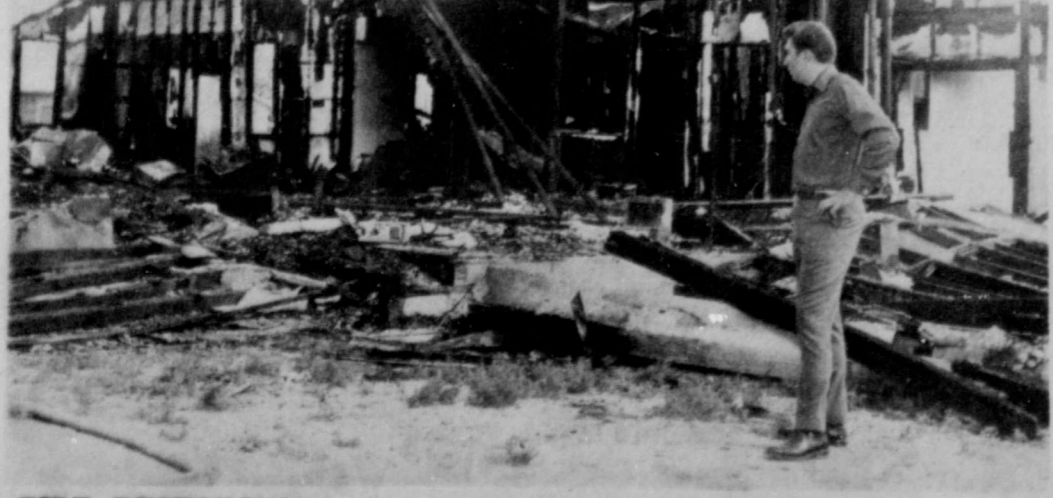
FIRE DESTRUCTION...Assembly of God Pastor W.G. Lillard views destruction after fire gutted the building early Monday morning. (Staff Photo)
