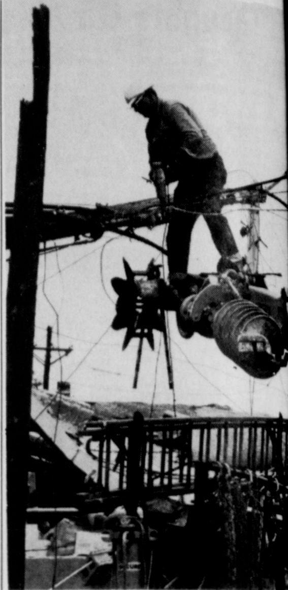
CUTTING TELEPHONE CABLE loose from er lines after killer tornado struck Lubbock May 11 was major job for Dave Gamble, Southwestern Bell Telephone Company from Plainview. Crews from throughout Texas began arriving on the scene within 24 hours. Service was restored to normal by last week.
