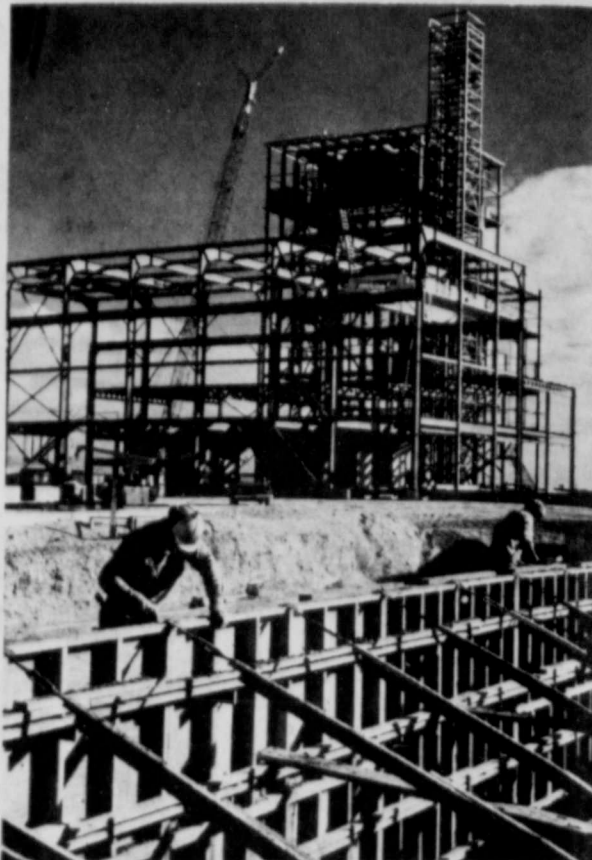
A MAJOR INVESTMENT in Southwestern Service Company's 1970 construction program, the Clifford B. Jones Generating Station being constructed on the South Plains near Lubbock, electric company plans to invest more than $25,000,000 in plant and equipment in 1970.
