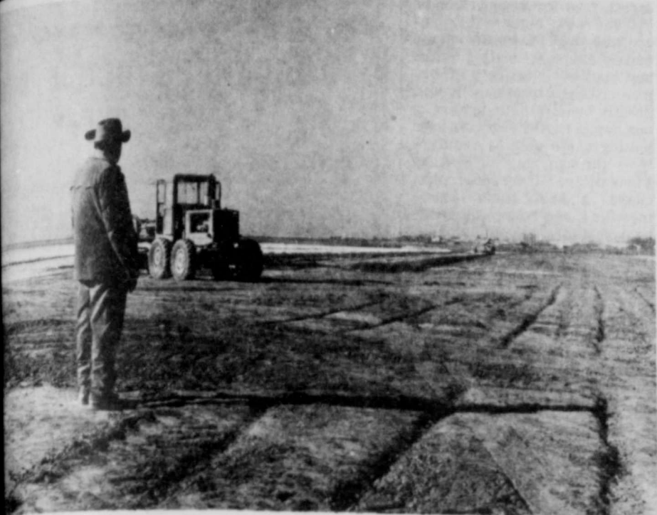
ACTIVITY IN SOUTHEAST FLOYDADA... as work begins on paving five acres for auto transport company unloading and storage. (Staff Photo)
