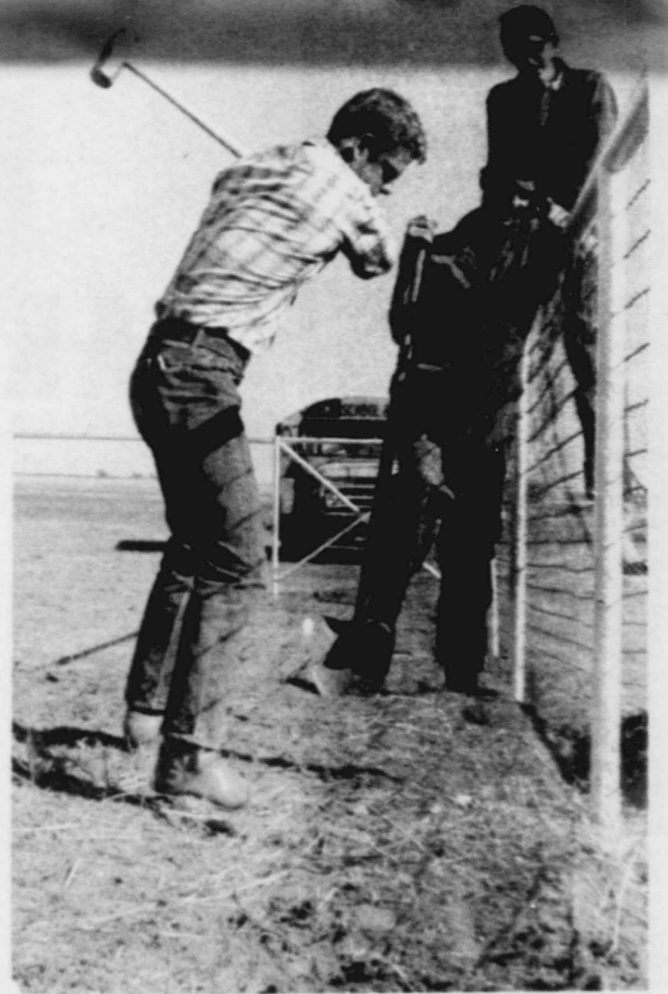
BUILD STOCK PENS - In November, the Floydada FFA Chapter built stock pens on the Rodeo grounds in southeast Floydada. Pictured above are (from left to right) Dayne Golightly, Sammy DeLeon and Mike Carroll. (Staff Photo)
