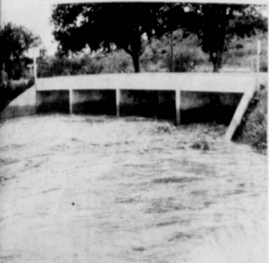
EVER... note water line on bridge
