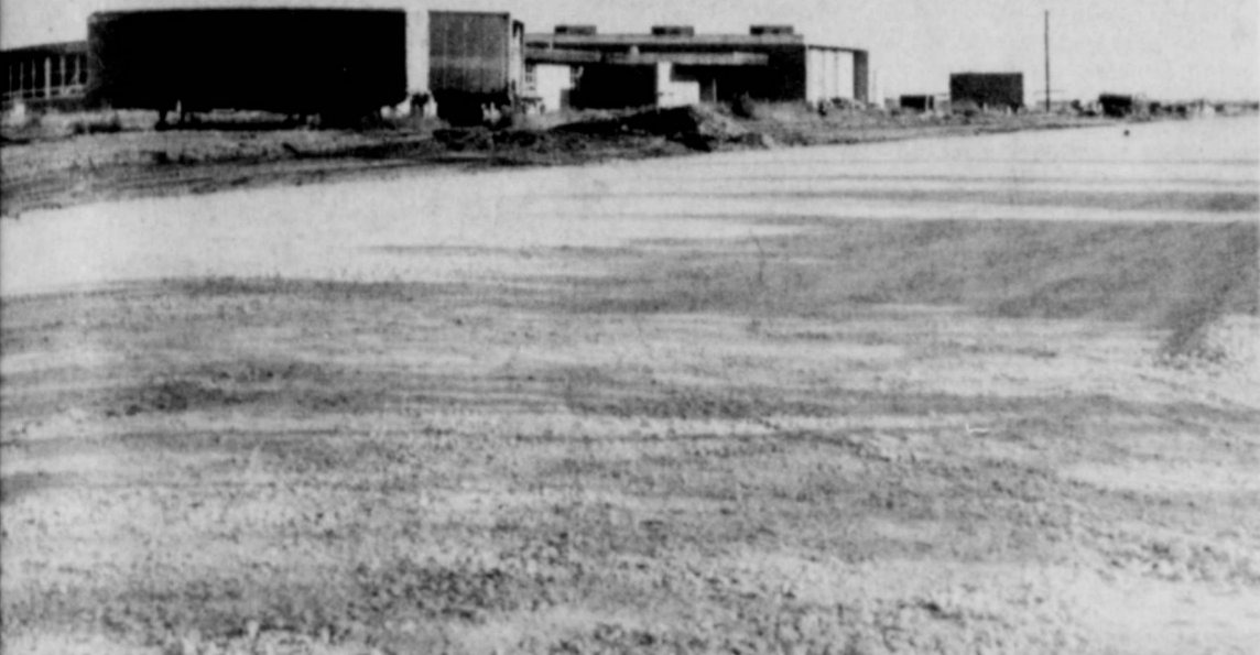
PROGRESS - three and a half blocks are being paved in front of the new Duncan Elementary School east Floydada. Other paving activity includes a block on Marivena, three blocks in the Steen addition and the new municipal airport. Contractor is High Plains Paving Inc. (Staff Photo)
