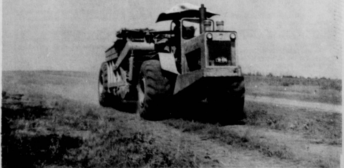
AND NOW BACK TO THE AIRPORT! - at last work begins on the construction of Floydada's new airport. Contractor Bryan-Hoffman of
