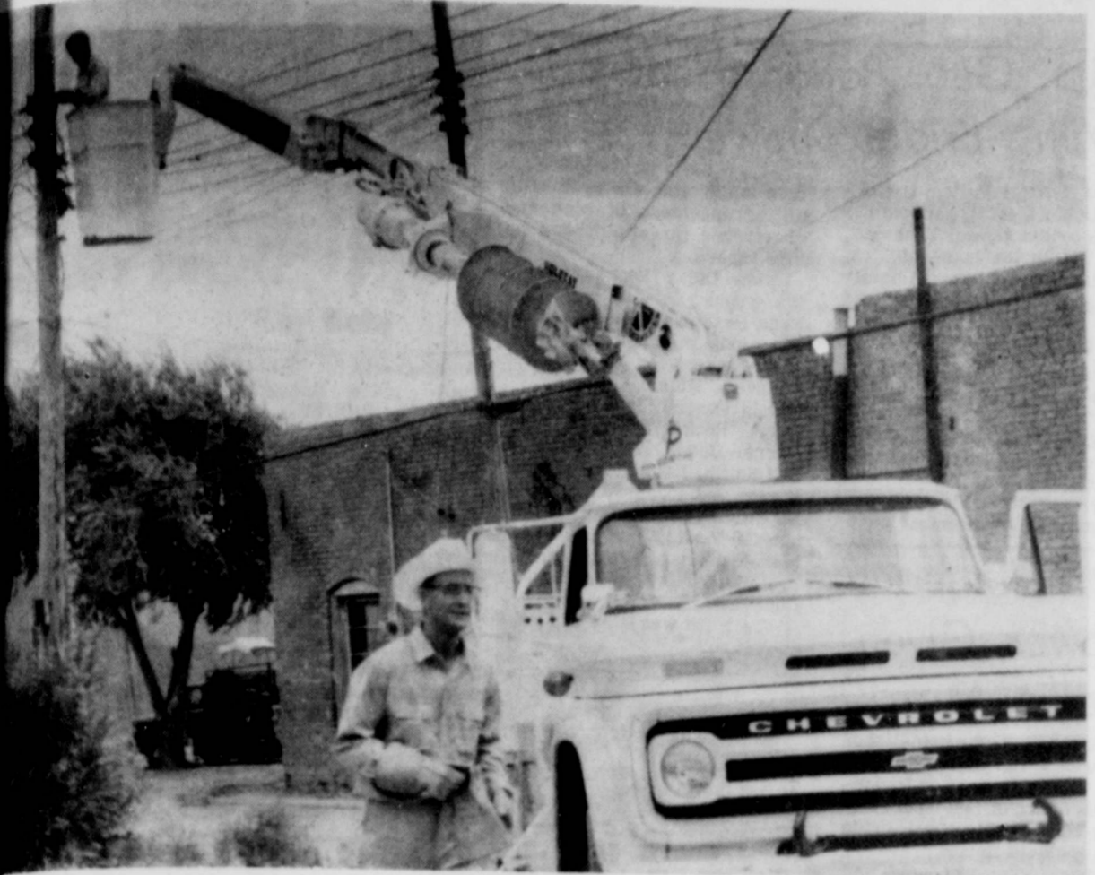
The newest addition to the city's pole cat that is shown above. Insulated so that danger of injury in the bucket is cut to a minimum.
