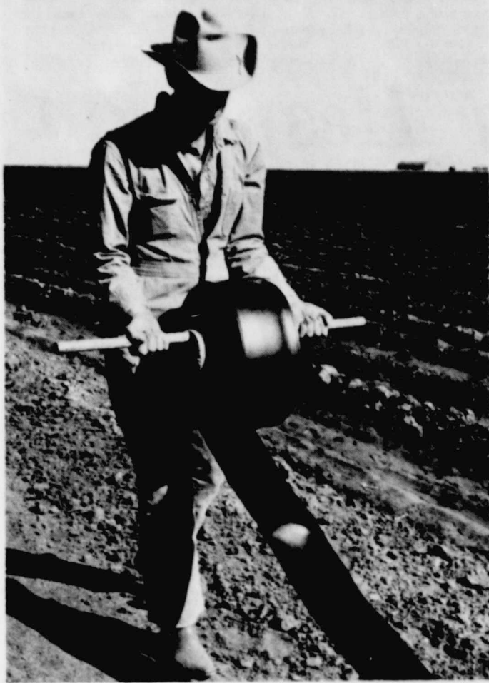
BU TUF TUBING - This photograph was made on a Plains area farm during installation of the dramatically-new Bu-Tuf portable irrigation system recently introduced in this area. The Bu-Tuf system is made of thin-wall plastic tubing with diameters ranging from 4 1/4", shown here, through 12 3/8". The system gives the farm operator total flexibility and permits changing irrigation layouts as needed. With the system, the portion of the ditch used to transport water to the point of irrigation can be eliminated, greatly reducing the costly losses due to seepage and evaporation.
