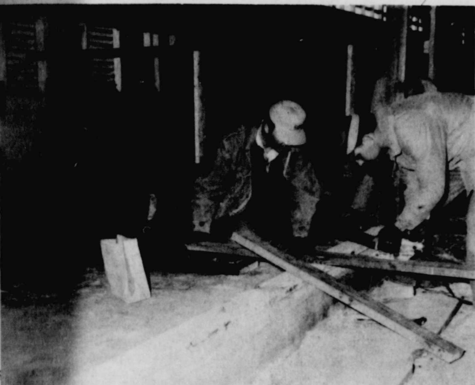
RACK--Members of the Floydada Chamber spent several hours preparing, pouring concrete, and walls to build a new wash rack
