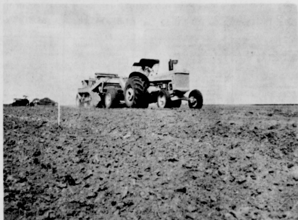
LAND LEVELLING - Pictured above is a land levelling operation on the K. E. Probasco farm 4 miles north of Barwise. Uneven and steep slope is being brought to a uniform grade of .2 foot fall per 100 feet by making cuts and fills according to a design developed by the Soil Conservation Service. (SCS Photo)
