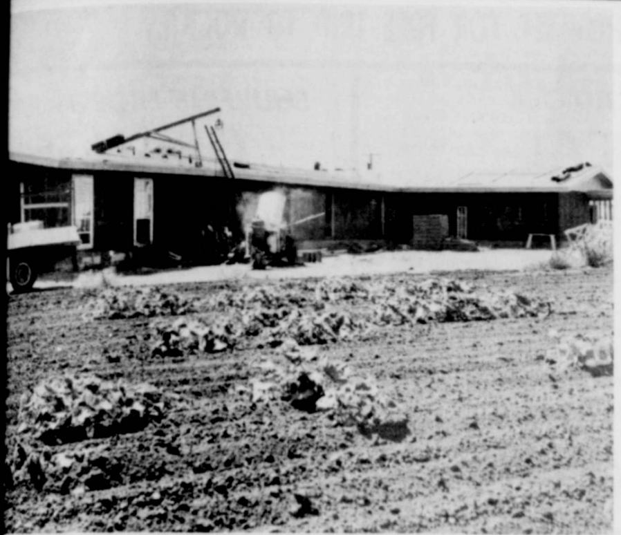
MANOR CONVALESCENT CENTRAL—walls are up on the three wing unit being constructed southwest of Floydada, and west of the Ralls Highway. (Staff Photo)
