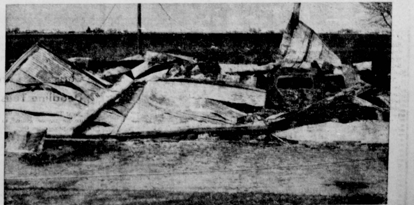
TOTAL LOSS — The scene above is what is left of a metal building belonging to V. D. Turner on the Matador Highway. The building burned to the ground. Inside the building were four cars, 2 irrigation engines, a boat and trailer, a camper and an undetermined amount of shop equipment.
