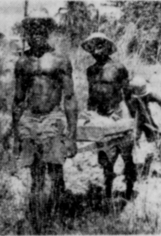
Haitian workers carry rock on a "bouret" to construct a roadway which connects remote villages in Haiti to a main thoroughfare. The men were paid for their labor in food — some of it beans from CROP.
