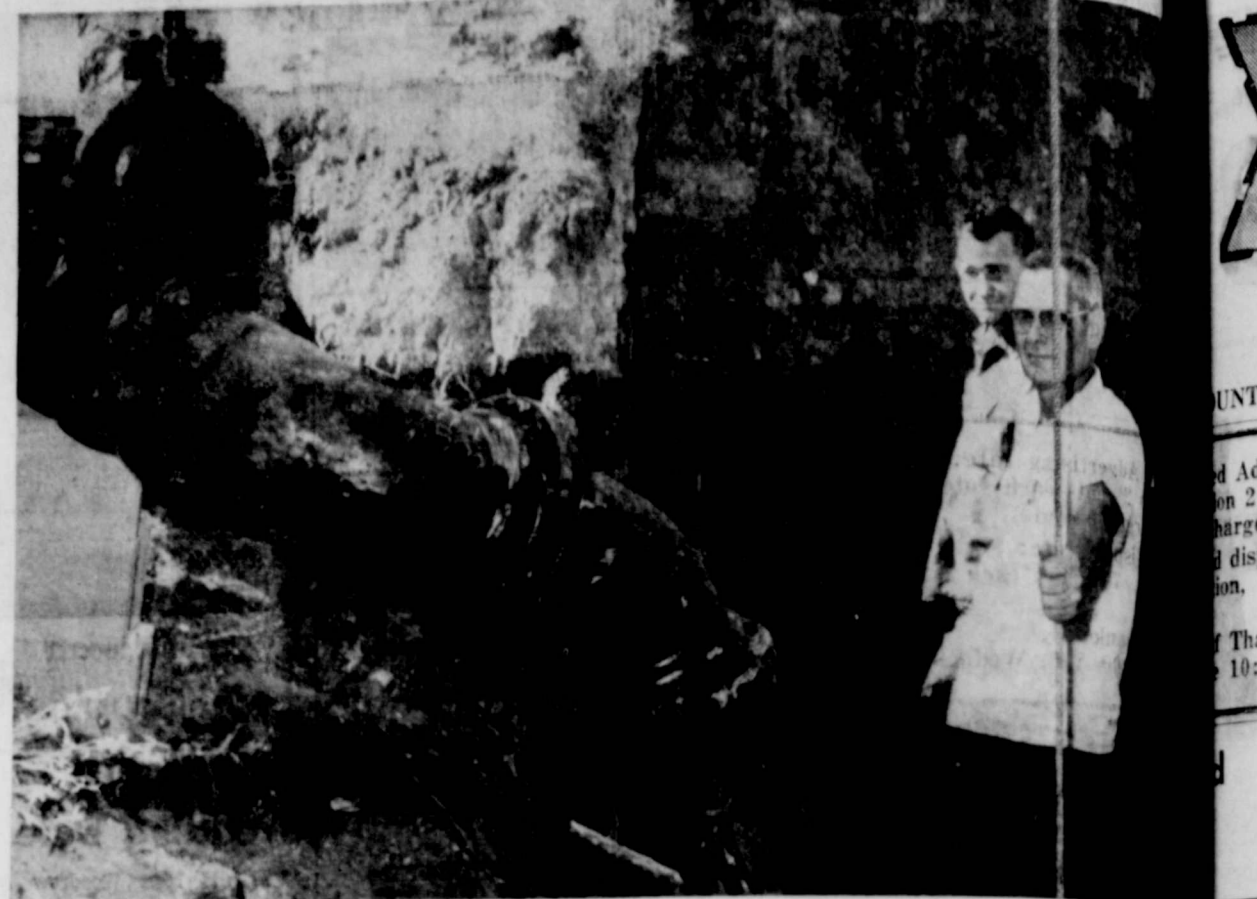
CHLORINATION SYSTEM — Bobby Welborn, rear and Harold Huggins are shown connecting the new chlorination system onto the city's main storage tank on the Ralls Highway. The
