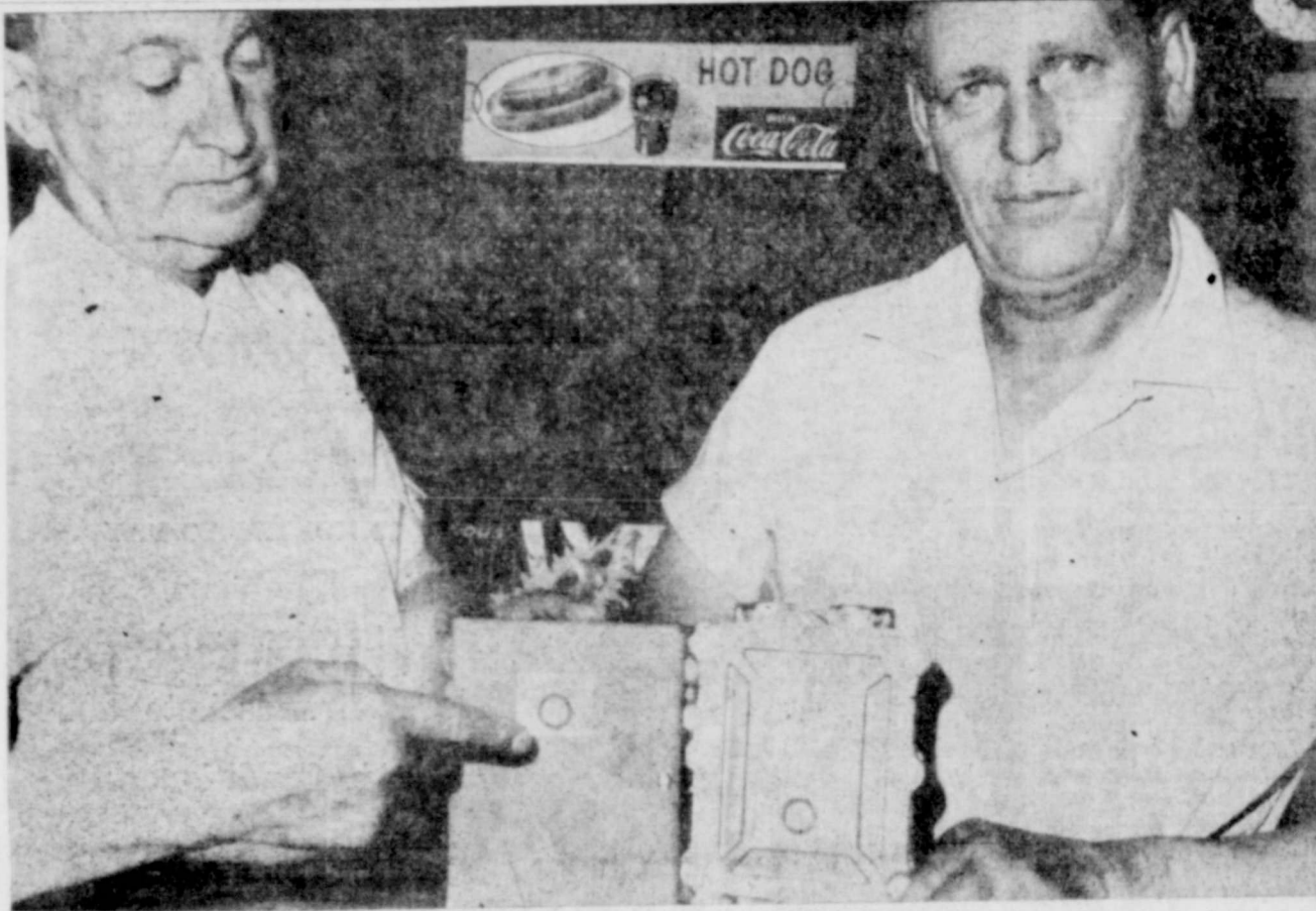
INSTANT HOT WATER FROM THIS LITTLE GADGET ... was found to be true after it was installed in the Palace Theatre rest room. It's a Jetomic and gives you hot water at the turn of the tap. Royace Maddox, left, Jack Lackey, right and Jack Deakins, manager of the Theatre not pictured, are distributors for the Jetomic in this area. (See Story elsewhere) (Staff Photo)
