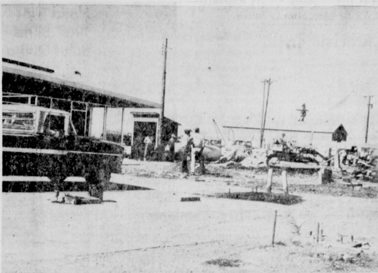
OUT WITH THE OLD... IN WITH THE NEW! A bulldozer clears out the old service station as a modern new station and restaurant
