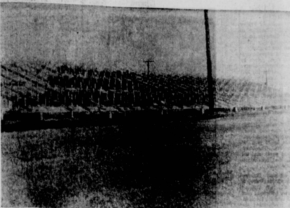
BRAND NEW STANDS GOING UP . . . stands for the entire west side of the Floydada football stadium are going up and the steel framework is pictured above. Pressbox and seats are yet to be built.
