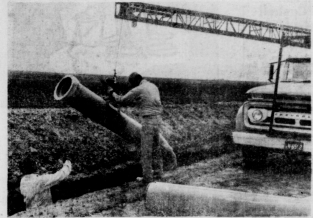
$2500.00 cost share is available for irrigation pipelines under GPCP. Cost share rate is 50%. All sizes and types of irrigation pipelines are included in the GPCP handbook. Shown is rubber gasket type pipeline being installed.
