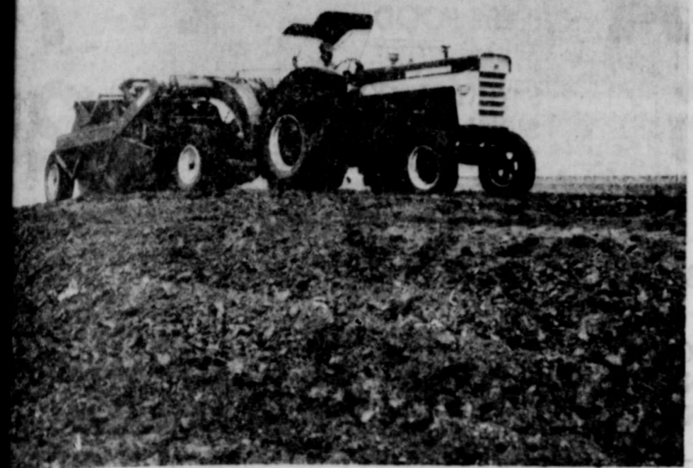
Leveling is included in the GPCP handbook with cost share rate of 50%. Land leveling on Gene Probasco farm. A uniform grade must be installed for assistance.
