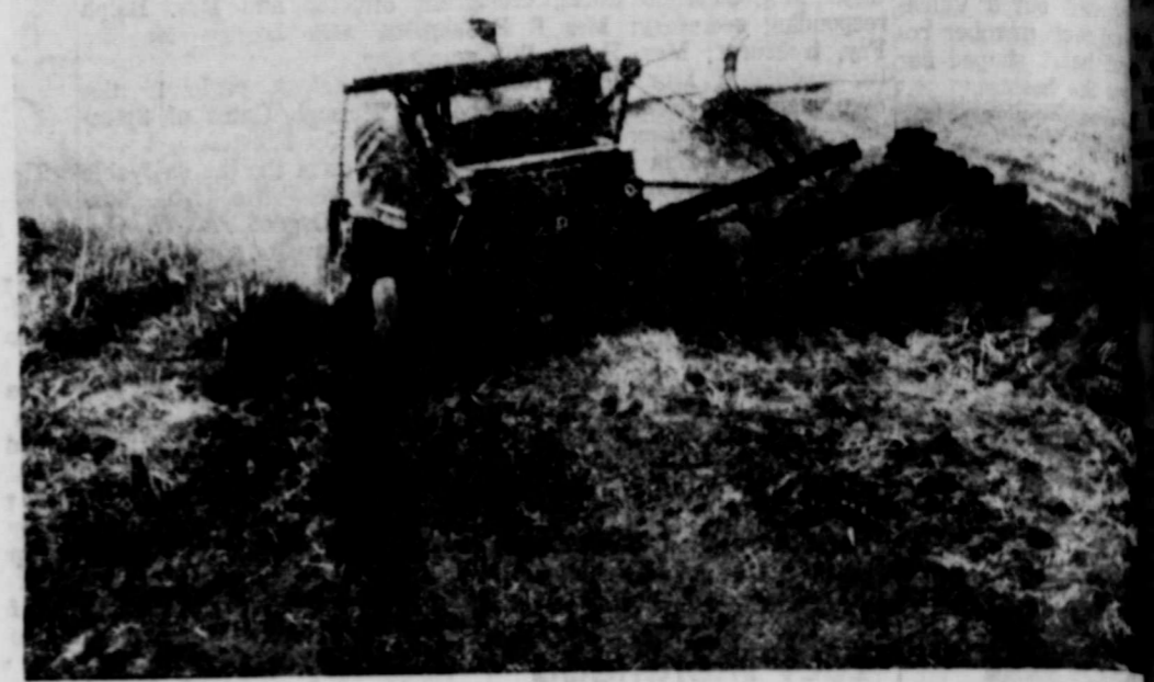
Terrace systems may be constructed with an elevating terracing machine as shown in this picture. Level closed-end terraces constructed in the Floyd County Soil Conservation District are wide enough that four row equipment may be operated on them without slippage after the terraces have had a chance to settle.
