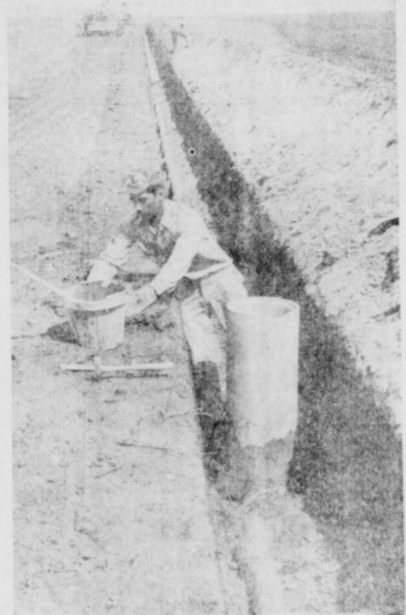
Installation of valve on a rubber gasket type pipeline on the Joe Dunn farm south of Floydada. This line will provide water to a Midland bermuda grass pasture. Cost-share of 50 percent on irrigation pipelines is available to those carrying out a complete conservation plan under the Great Plains Conservation Program.
