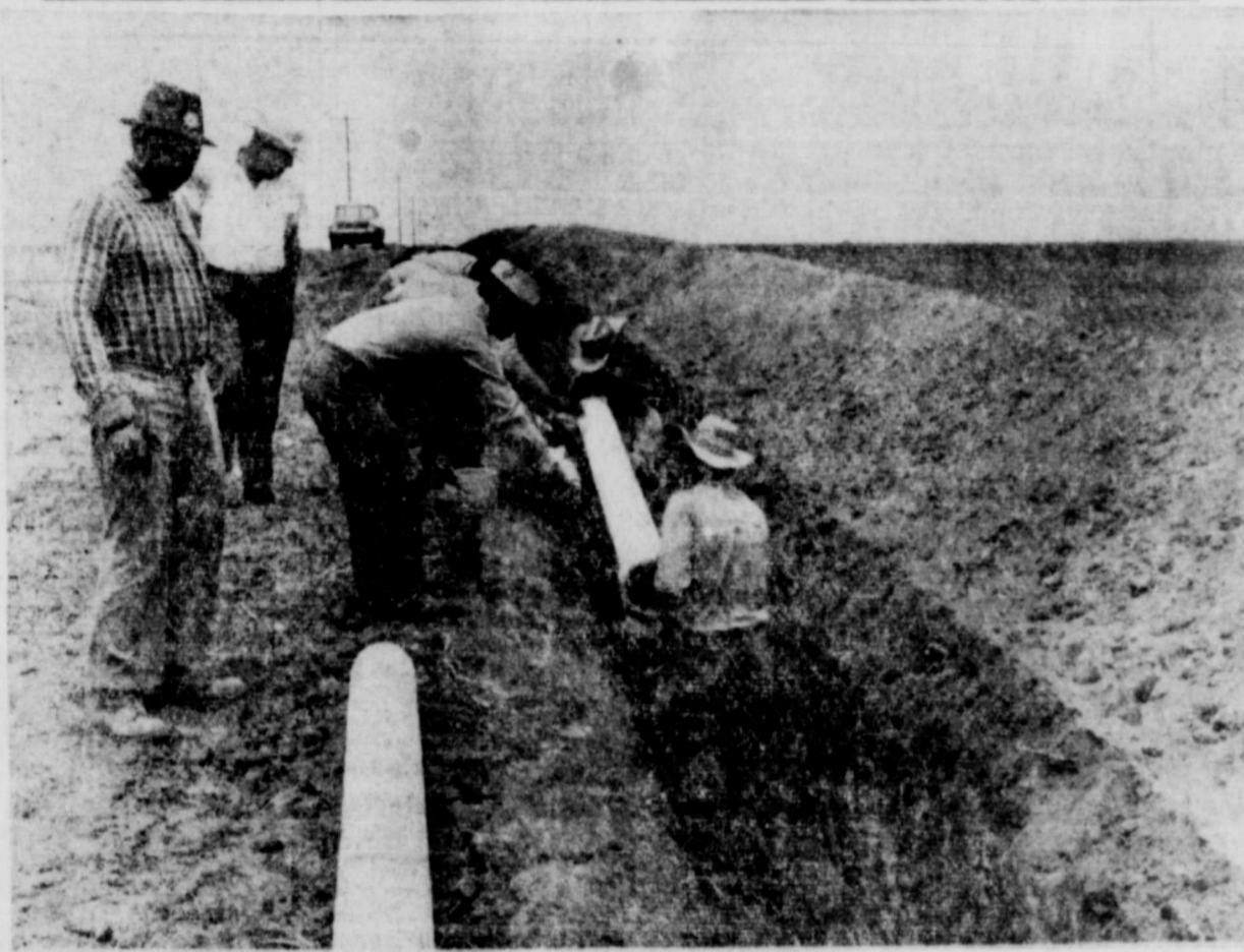
Cement asbestos pipeline being installed on Leroy Durham's farm. This is a part of a sprinkler system for irrigation of a Bermuda grass pasture.
