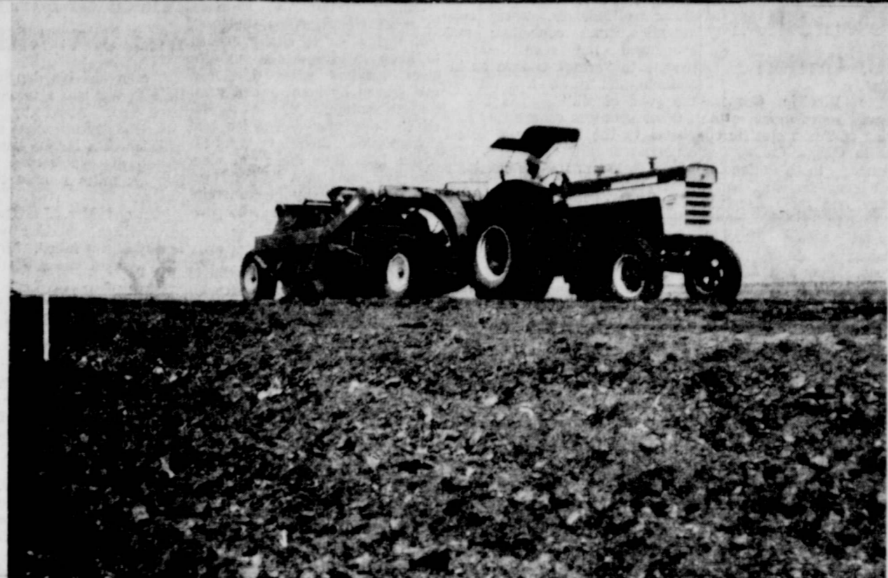
PHOTO SHOWS construction of a diversion terrace on W. A. Cox farm northwest of Floydada being built under the Great Plains Conservation Program. Terraces of this type are suited both on irrigated and dryland farms. They are used to break up concentration of water, break up slopes, and heal gullies. The excess water is emptied out on grass. There are many farms in Floyd County where this practice is needed. The GPCP will pay 70% of the cost of construction.
