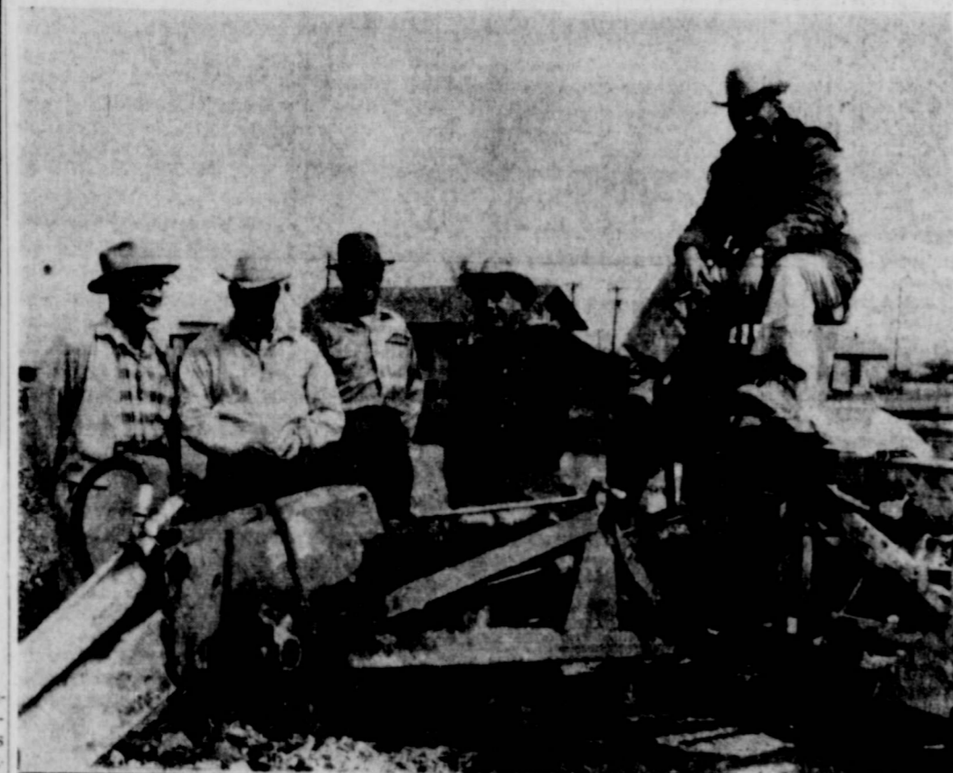
EXCAVATION BEGINS. Some of the members of the board of directors of Producers Cooperative Elevator Saturday watched the beginning of excavation for their new flat storage building on East Missouri St. The big power shovel was excavating a hole seven feet deep, five feet wide and 210 feet long. Several such will be used for aeration tunnels, making when finished 4 x 6 concrete tunnels the length of the building. Here, left to right, are manager Roy Jones, Director John K. West, President Tom Porter, Vice President Roy Hale, and subcontractor Charlie Richardson. (Staff photo)
