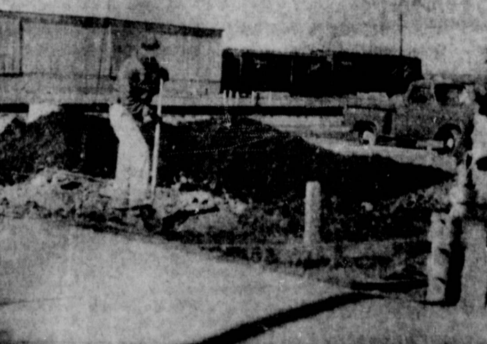
STRINGER CONSTRUCTION CREW are seen above as they start work building a new office for Lon Davis Grain Co., on East Houston Street. Mr. Davis has temporary quarters in the Morckel Co. building until the new office is completed.
