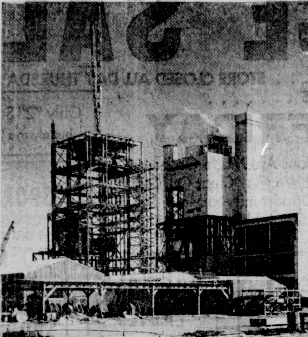
One project in Southwestern Public Service Company's $22,000,000 improvement program for 1961, will be continued work on Nichols Station, northeast of Amarillo. The generating capability of the plant is being doubled.
