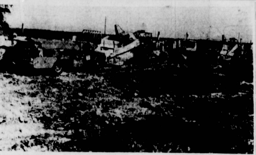
ROAD BUILDERS on Highway 62 this week had begun to level off for their half a million dollar job of re-building the highway from the wye in southwest Floydada to the Crosby County line. Two weeks ago they "lit" ready to work, but the big machinery, part of which is shown here, sat idle while the water receded. Two big lakes are being drained this week by the use of lake pumps and drainage ditches. Strain Bros., a San Angelo concern, has the contract. (Hesperian staff photo and engraving)
