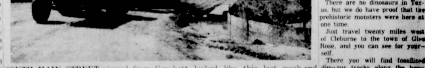
SOUTH MAIN STREET viewed from Crockett looked like this last week-end when the Thomason dirt moving crew got back on the job after three weeks of starts and stops. Note water in the gutters, occasioned by breaks in the water lines. Half a dozen such minor repair jobs were still on water superintendent's list this week, in addition to bigger jobs (of lowering mains) the water department encountered when the paving work began. The outlay on the part of the city has been in the thousands of dollars. (Staff photo and engraving).
