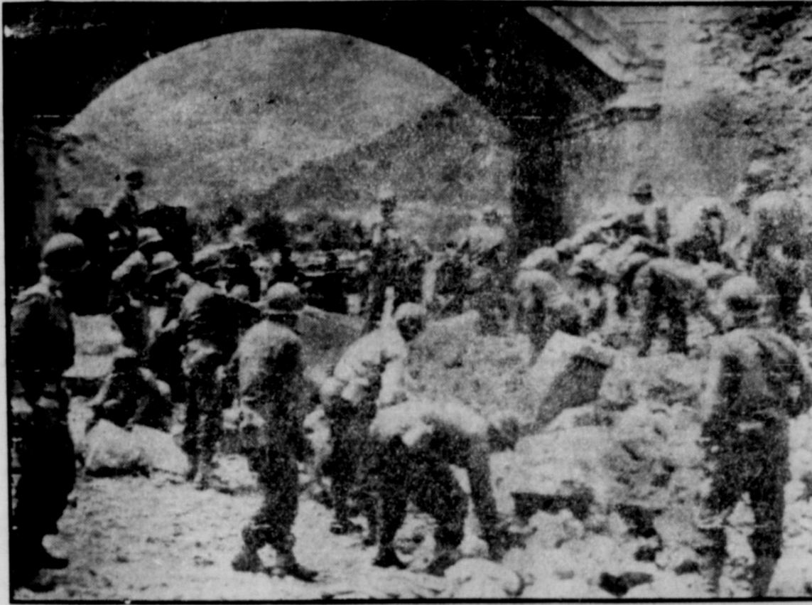
Near Itri, Italy, American engineers clear the blasted Appian Way where it passes beneath a railroad viaduct. This forerunner of the modern super-highway was begun in 312 B. C. by Appius Claudius Caecus the Censor. Succeeding emperors extended it until it terminated at Brundisium (Brindisi) near the Adriatic coast about 244 B. C., furnishing a trade route to the east. Originally it was a two-lane, stone-surfaced highway 15.5 feet wide, 412 miles long. (Army Radio-Telephoto.)
