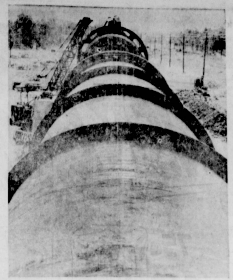
One of the world's largest single pieces of precision mechanized equipment, a 300-foot rotary kiln for the manufacture of cement, is being completed at the Texas Portland Cement Plant at Orange, Texas. The kiln will convert oyster shells into regular and special types of cement. Those responsible for engineering and constructing the facility have designated it as "the world's most modern cement plant".
