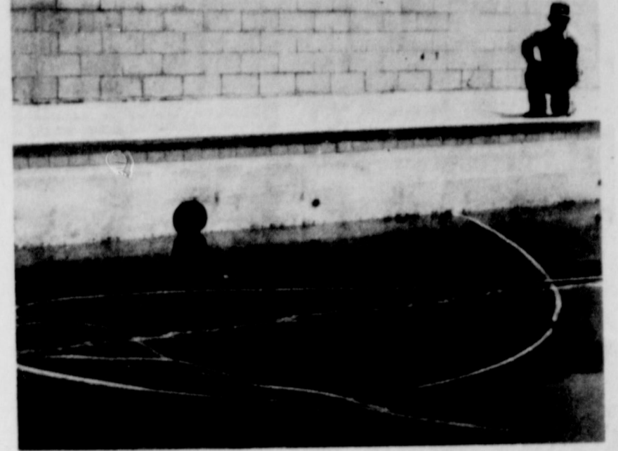
SURVEYS POOL... Larry Martin, City of Friona employee, surveys the mess which has collected at the Friona Municipal Swimming Pool, and must be rectified prior to the pool's opening. Martin is one of the city employees who is engaged in the refurbishing job underway
