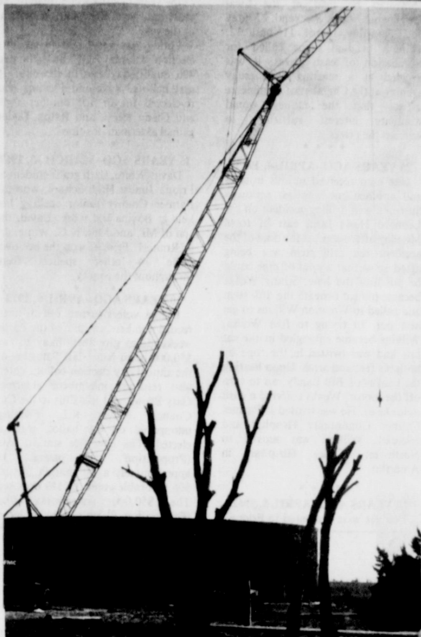
WORK UNDERWAY.... Construction work has been underway north of Friona on the million-gallon water storage tank for the City of Friona. Since the above photo was taken, another ten-foot section of the 32-foot high tank has been added. Bids on the pump station are slated to be awarded Monday, with completion of the $1 million project slated for August or September. Meantime, everyone in this area is ready for a good rain.
