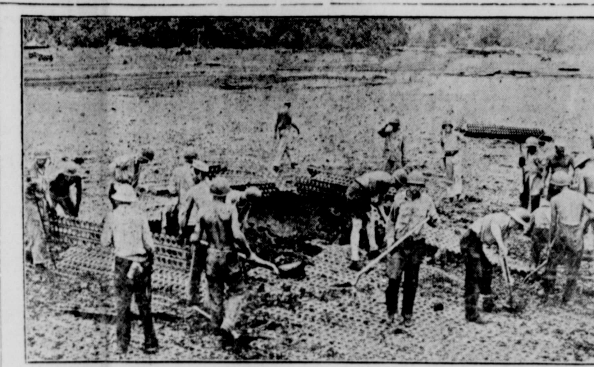
While We Eat Christmas Dinner.—This War department photo tells a story of lightning quick work a matter of minutes after enemy aircraft have bombed one of our air fields. Aviation engineers are shown on the job. Portable steel landing mats are being replaced. This scene was at Guadalcanal. It is being duplicated on all parts of the globe by our boys this week while we shop and make preparations for the Christmas feast.
