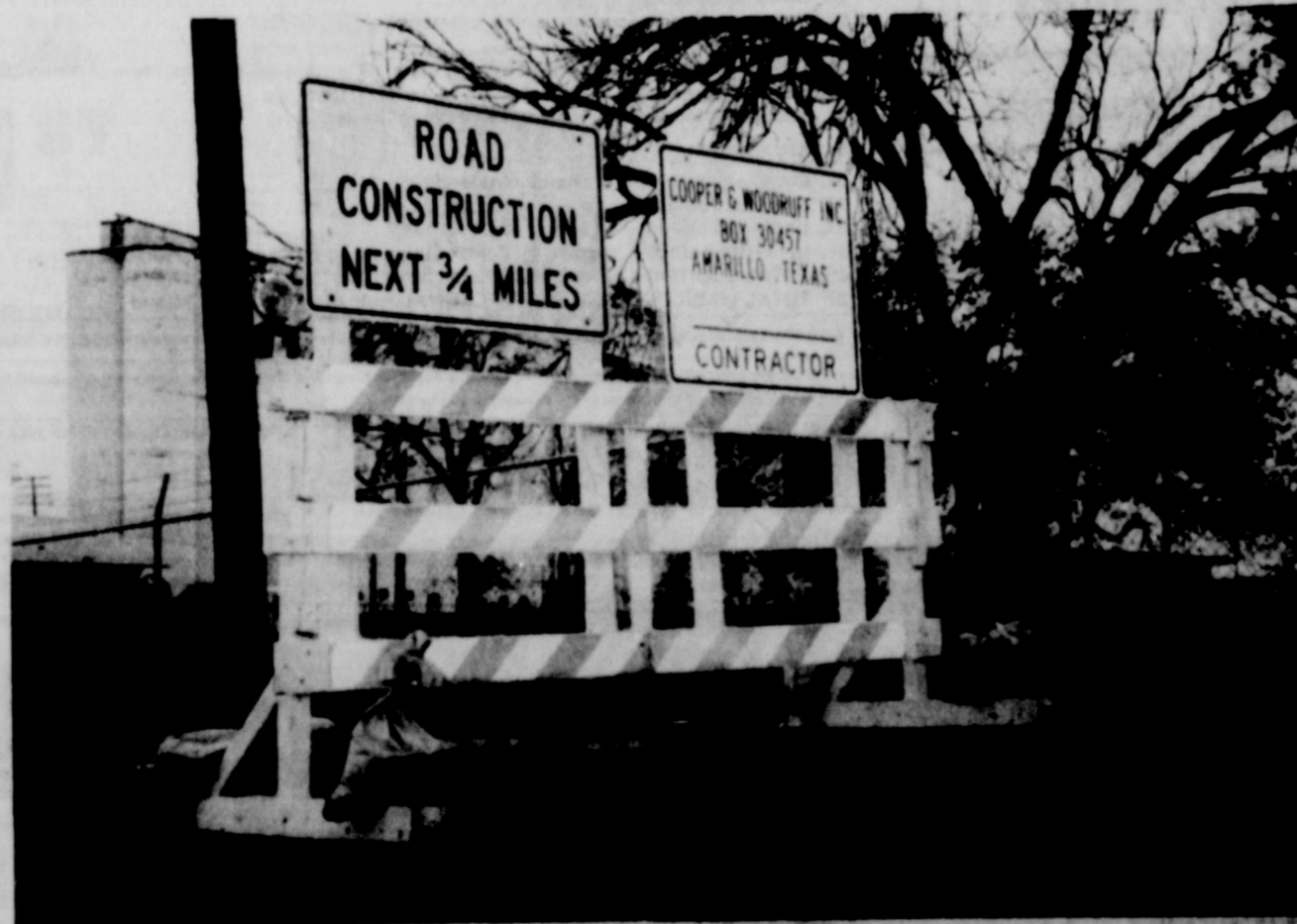
WORK BEGINS....One of the construction barricades on South Main Street is shown in the above photo. The barricade heralds the roadwork being done from the Santa Fe Railway crossing to the Frio Draw. A new bridge is to be constructed by the Texas Highway Department across the draw.
