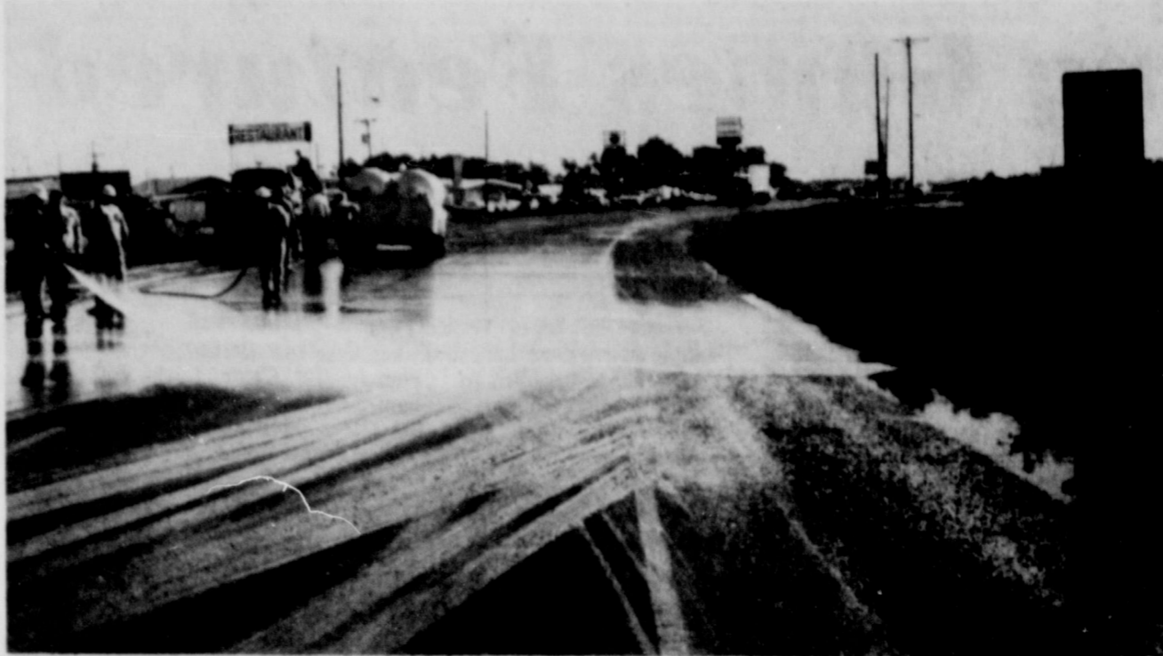
ROAD CLEARED.... Members of the Friona Fire Department were called to wash down a portion of Highway 60 on Thursday when a molasses truck ruptured and spilled onto the
