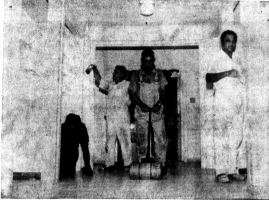
NEW FLOOR — Workmen putting in a new floor in the Goliad Junior High School band hall include Pedro Carrillo, J. C. Holguin, Jim Norman and Santiago Valencia. Much work is being done in the school system for maintenance and repair during the summer months.
