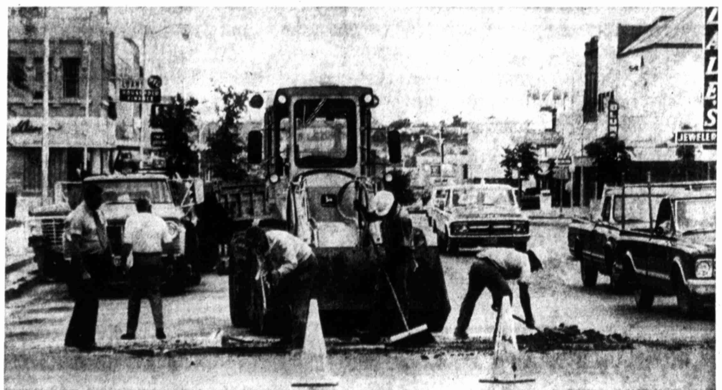
TEMPORARY INCONVENIENCE — Traffic was being stopped Wednesday morning at 4th and Main while the Texas Highway Department repaired a swell and crack in the pavement which
