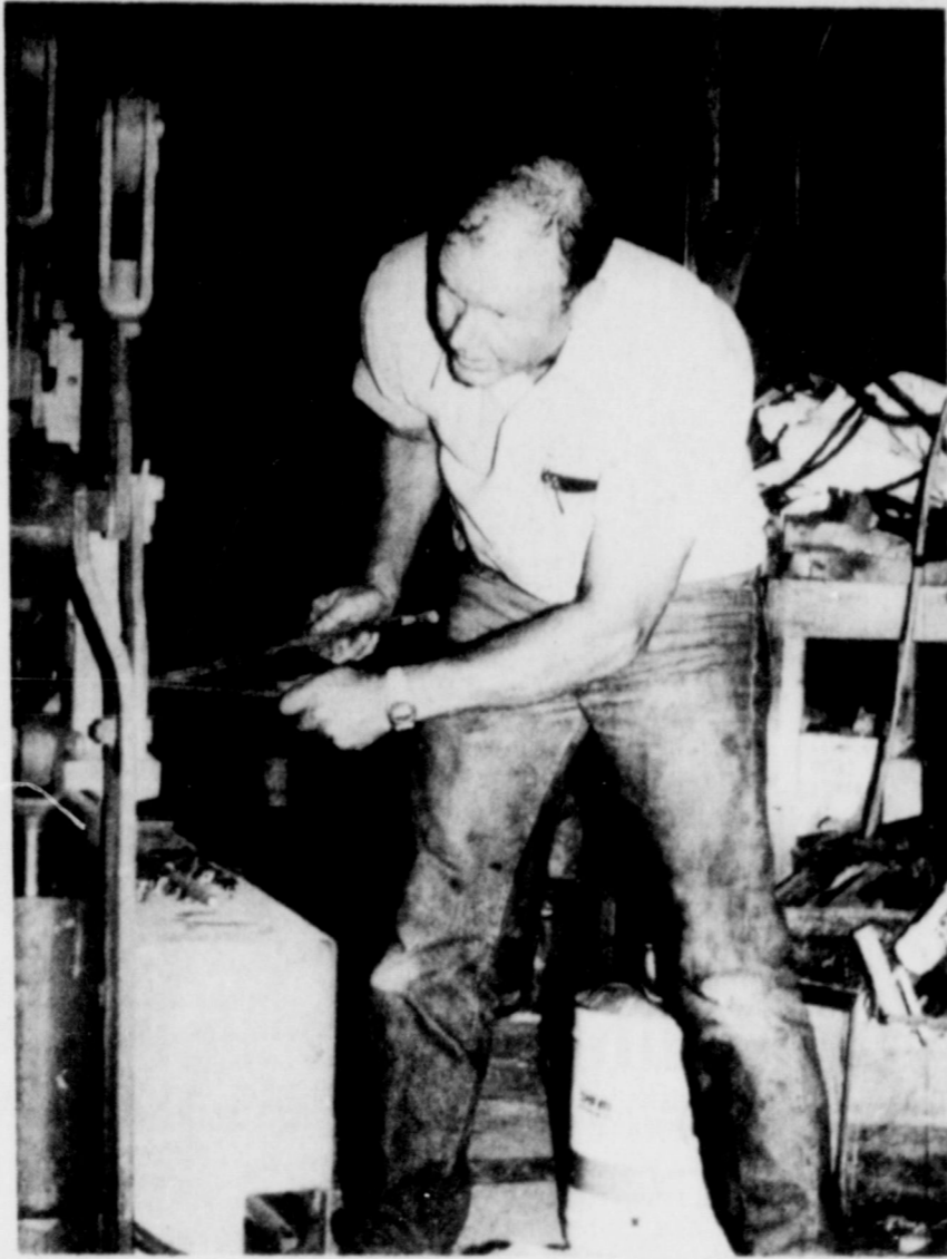
DELTON LEWELLEN is shown working on a pump which was installed on the new water well for the residents of Banderas, Mexico, last week. Lewellen was in charge of erecting a new church building for the Mexican community.
