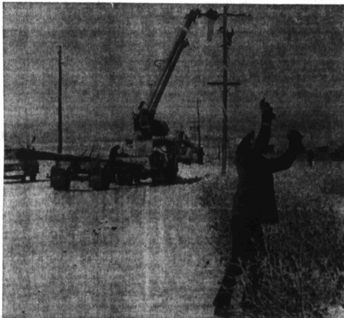
HOT LINE TO NOWHERE —The ice storm which descended upon the area last weekend played havoc with power lines north of Big Spring—an estimated 750 electric and telephone poles were felled in an area stretching from Big Spring to Tahoka. Power lines fell all over the country. Here, a lineman for Cap Rock Electric Co-Operative gingerly handles a broken wire and fellow workers toil to string new lines in the background.
