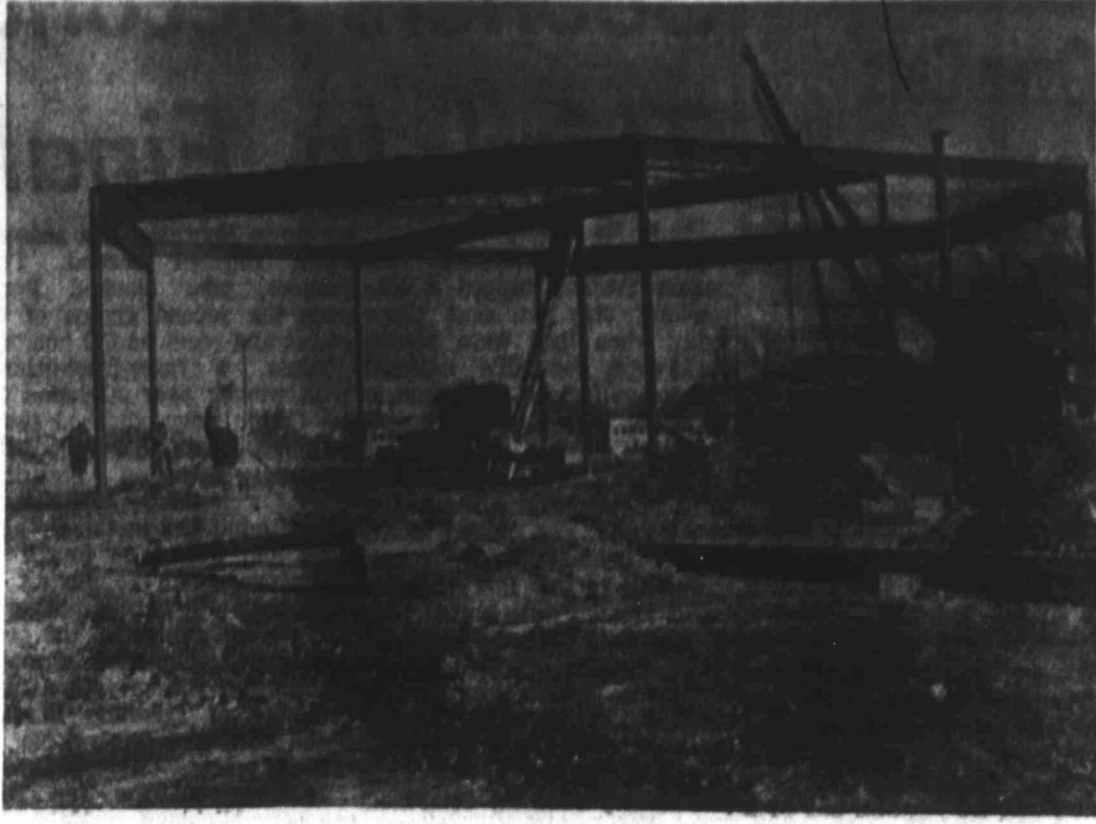
UNUSUAL SCHOOLS — Stanton is erecting a new elementary and junior high complex which includes two six-sided wings, with a traditional square building in between. Stanton also built an underground elementary school several years ago.
