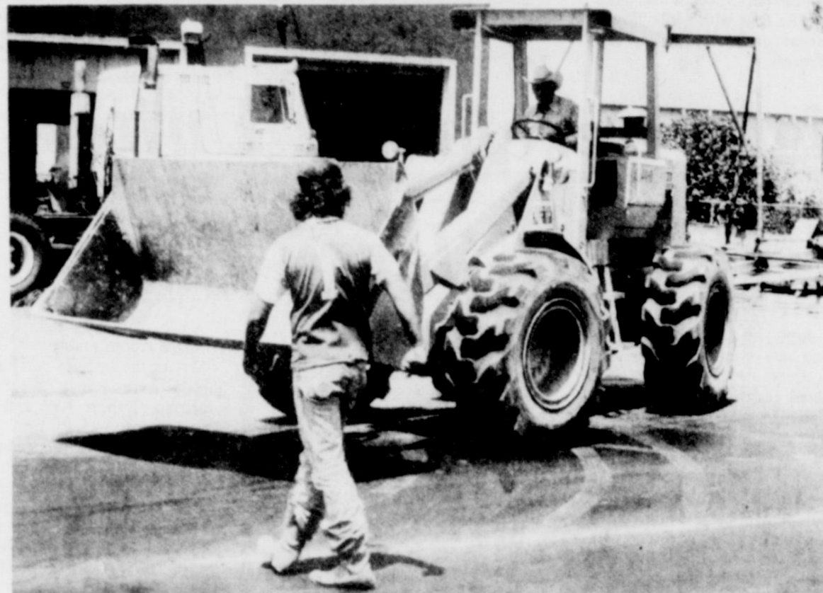
WORK BEGINS.... Construction work began this week on the highway project through Friona. The project will eliminate the medians on U.S. Highway 60 through Friona, and the
