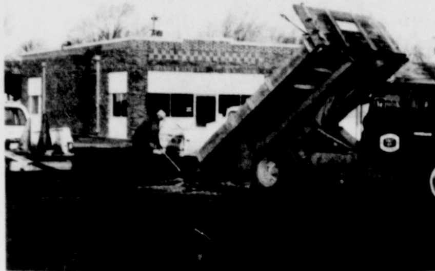
STREET WORK... City of Friona employees are shown making a street repair where a water line ruptured last week at Seventh and Main Streets. The sub-freezing weather was blamed for the break.
