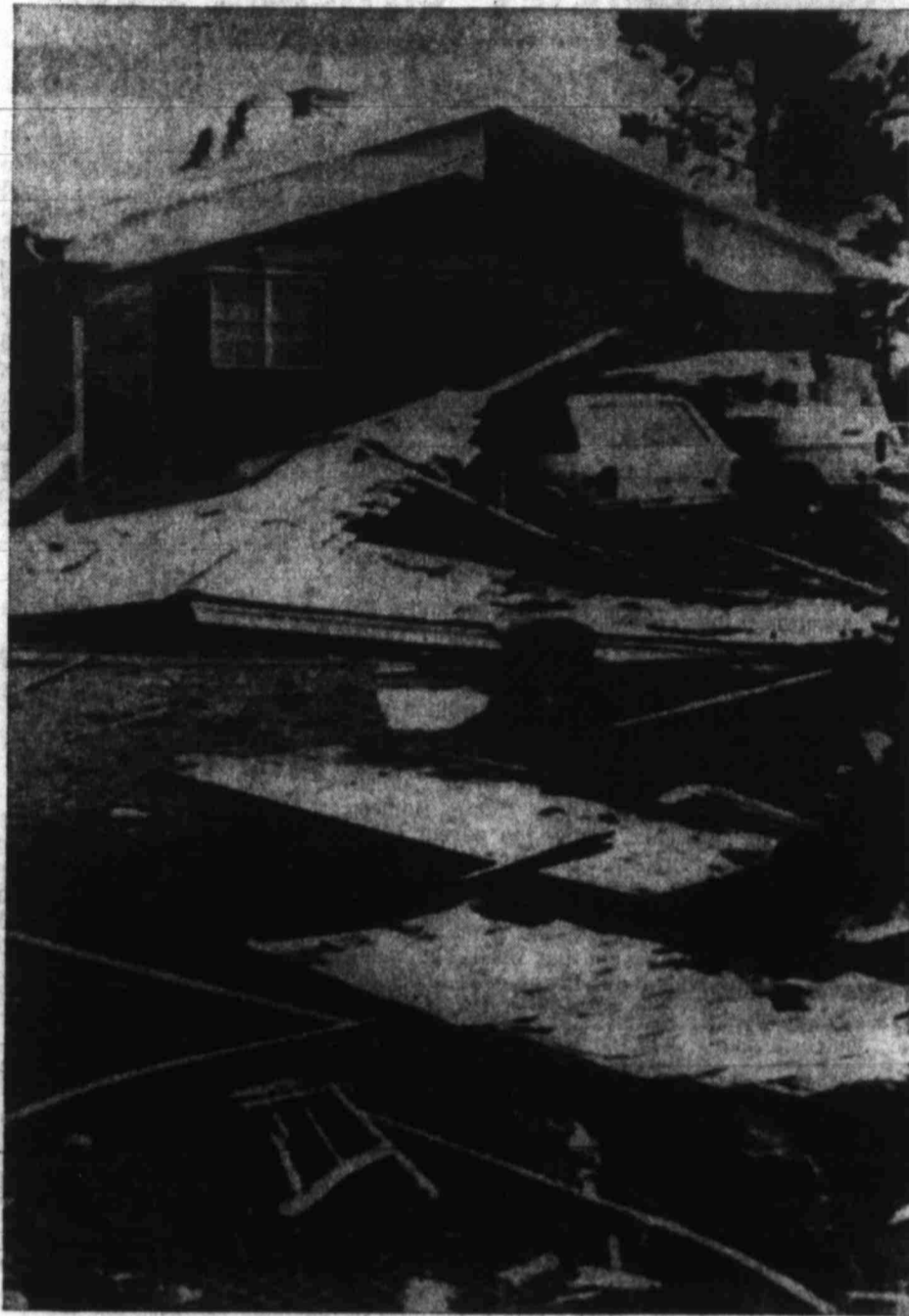
TORNADO DAMAGE — Heavy damage was done to the David Todd home when a tornado touched down early Sunday morning. The home is located near Marshall where the storm raked the area causing heavy damage but no reported injuries.
