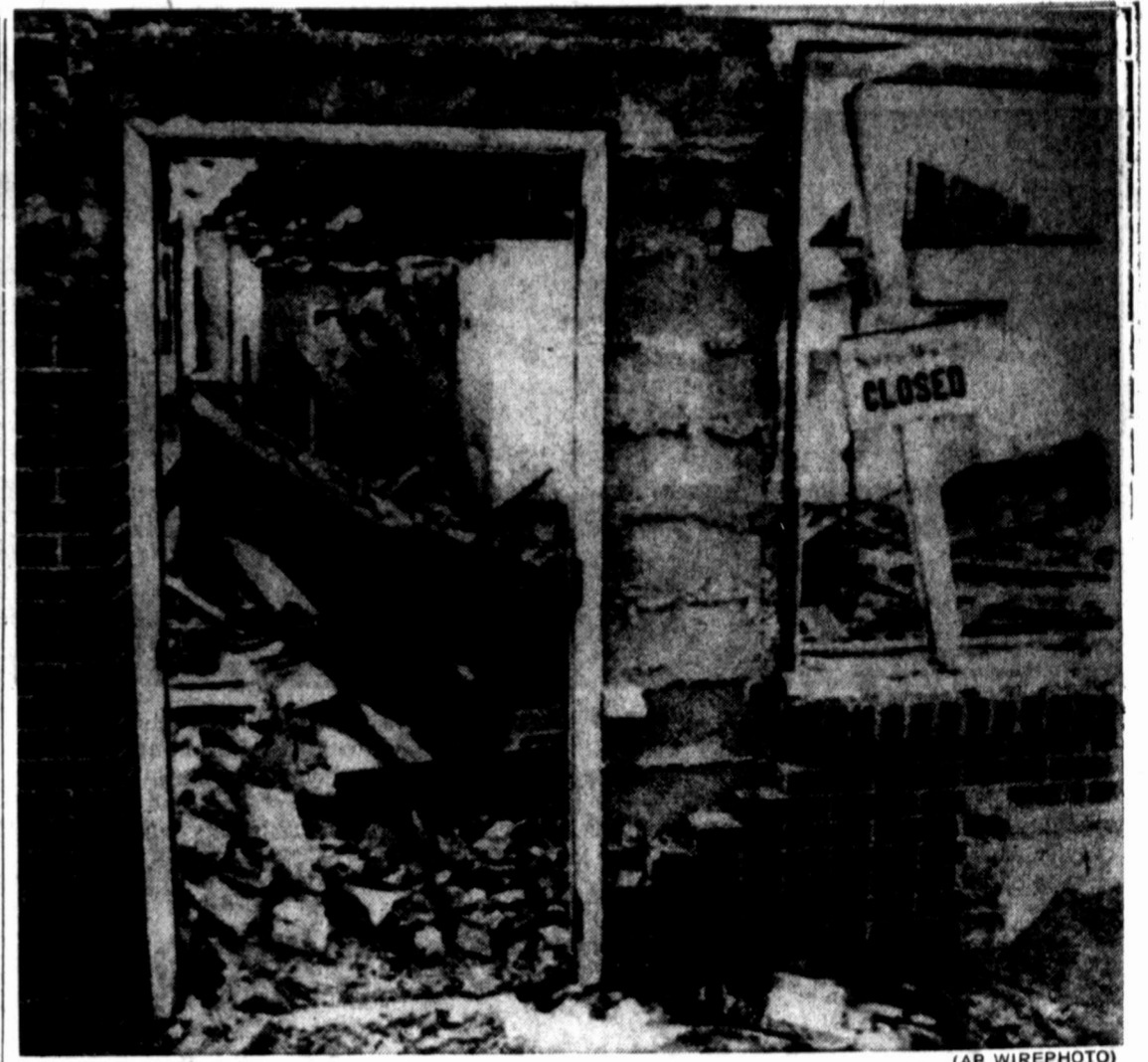
YOU GOTTA BE KIDDING! — The sign reads: "Sorry, We're Closed" but it looks as if this former restaurant at Limerick, Pa., near Pottstown, is wide open. A wag posted the sign as the restaurant was being demolished to make way for a bank expansion project next door.
